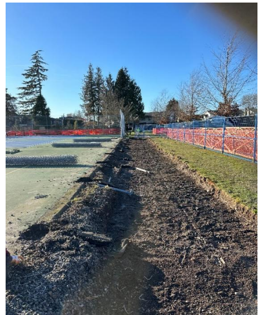
Figure 1-From North End of Courts looking West. Fence removed and trench dug for
