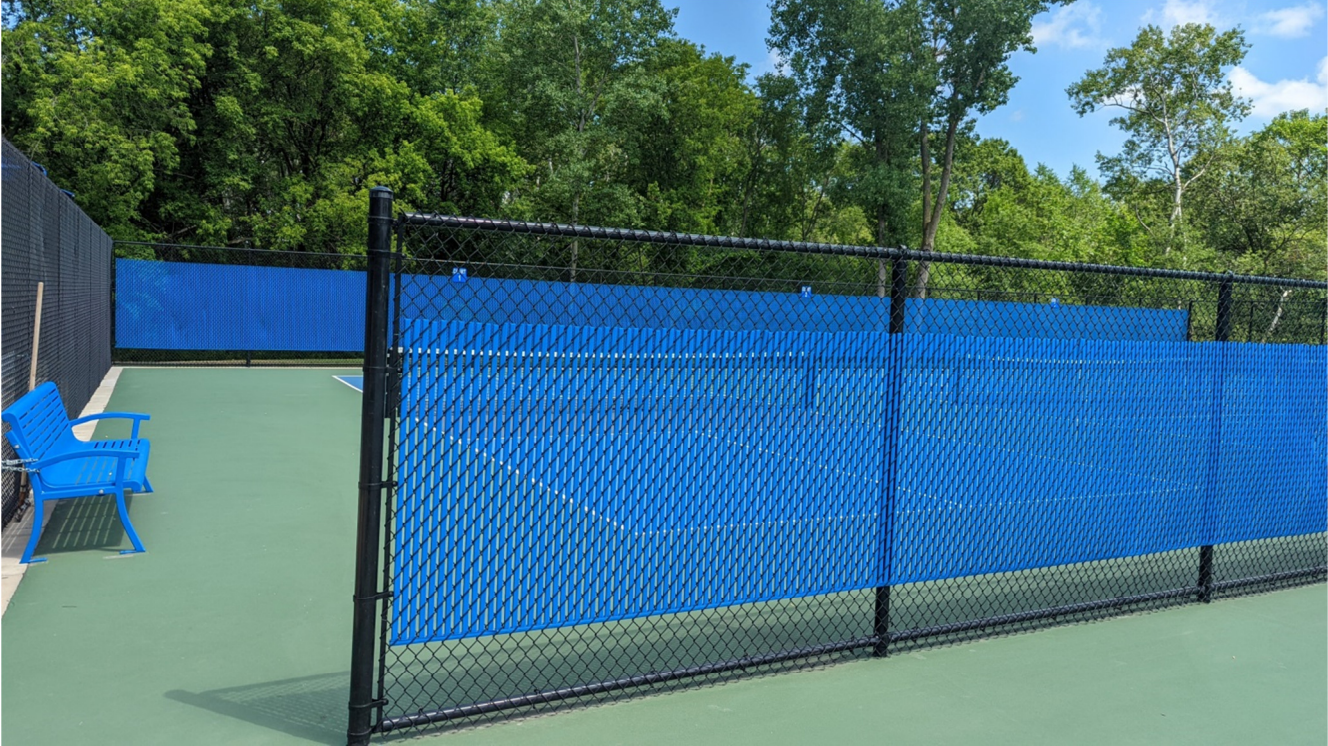
Photo 6, Rigid Windscreen Inserts in Perimeter and Intermediate Fencing
