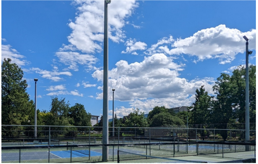
Photo 11, Pole-mounted High-efficiency Downlighting, Kamloops
